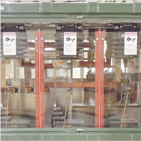
Separate phase cover barriers of 1/4" clear non-conductive Lexan for visual inspection
