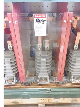
Separate phase cover barriers of 1/4" clear non-conductive Lexan for visual inspection
